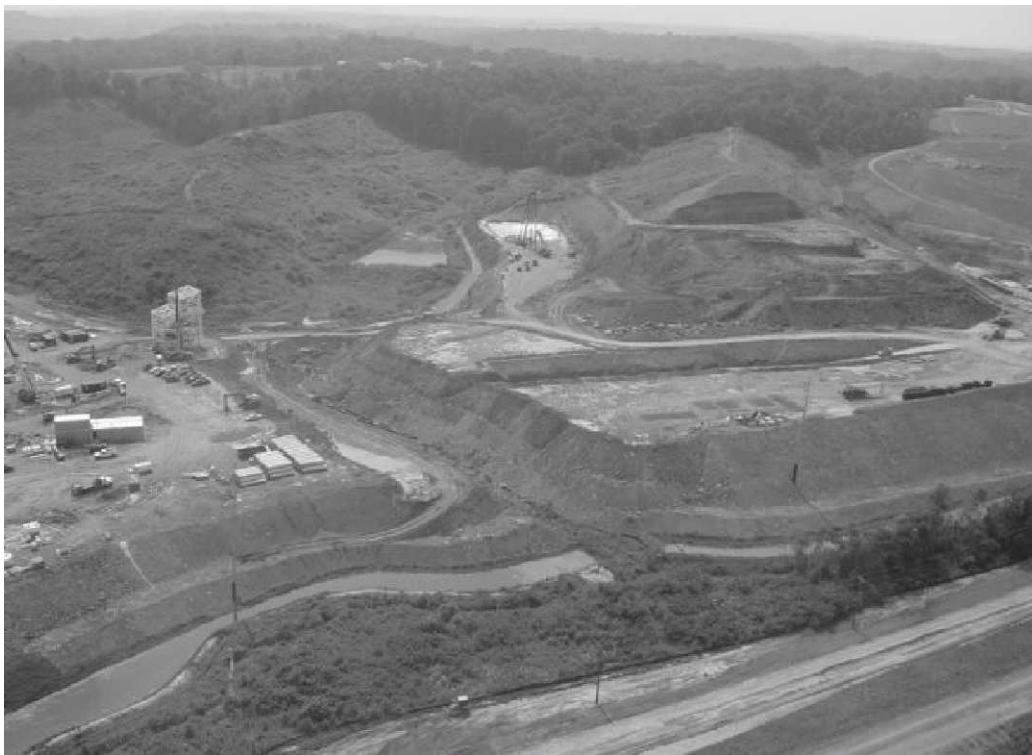
Construction of the Big River Mining, Broad Run Mine Complex in Mason County.
