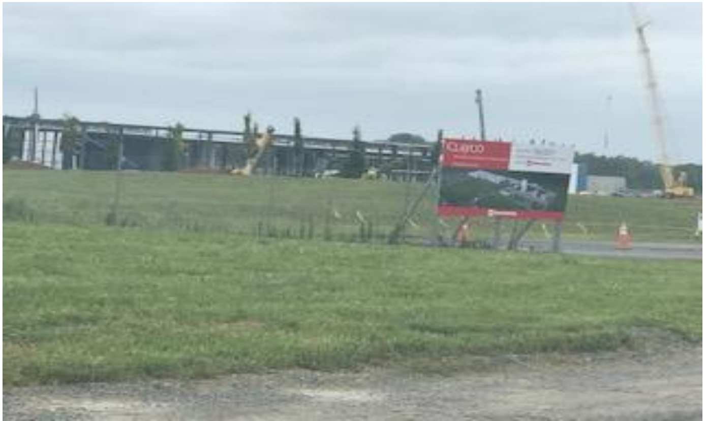
Rockwool Insulation Manufacturing Company
