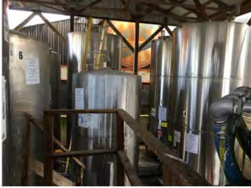
Secondary containment at a bulk facility.
