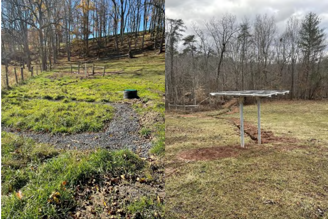
Spring Development/Solar Panel – Watering Systems
