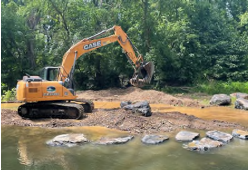
Boulder placement to enhance a stream in a watershed protection plan (WPP) priority basin.
