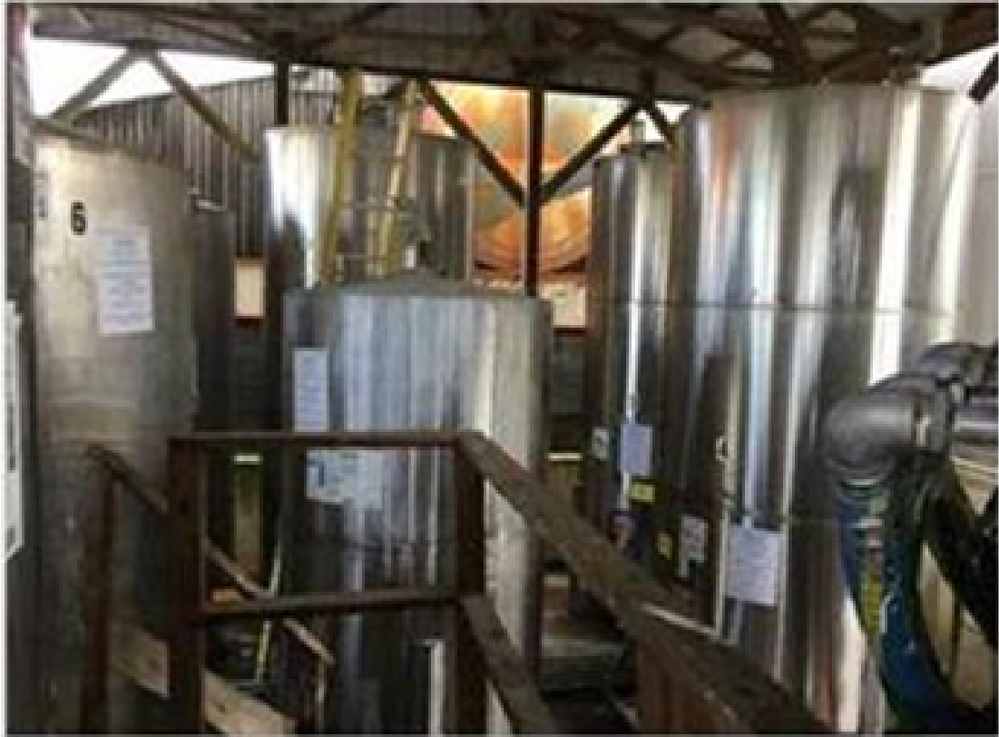
Secondary containment at a bulk facility.
