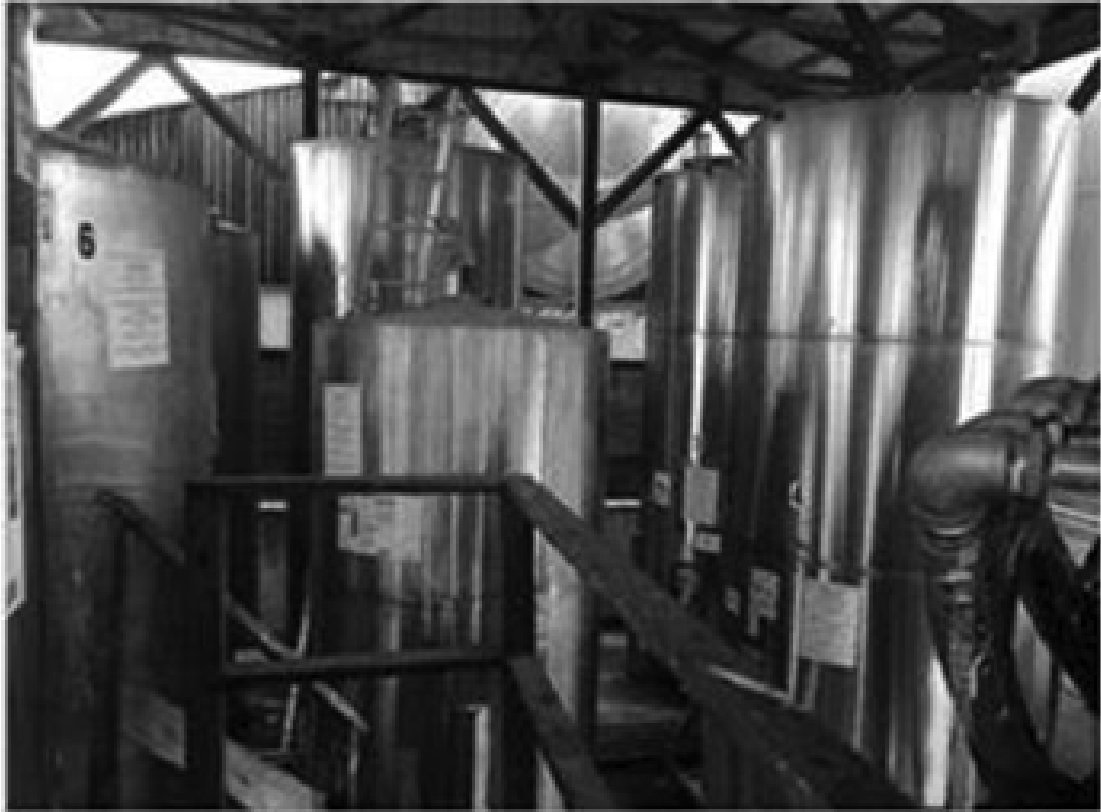
Secondary containment at a bulk facility.
