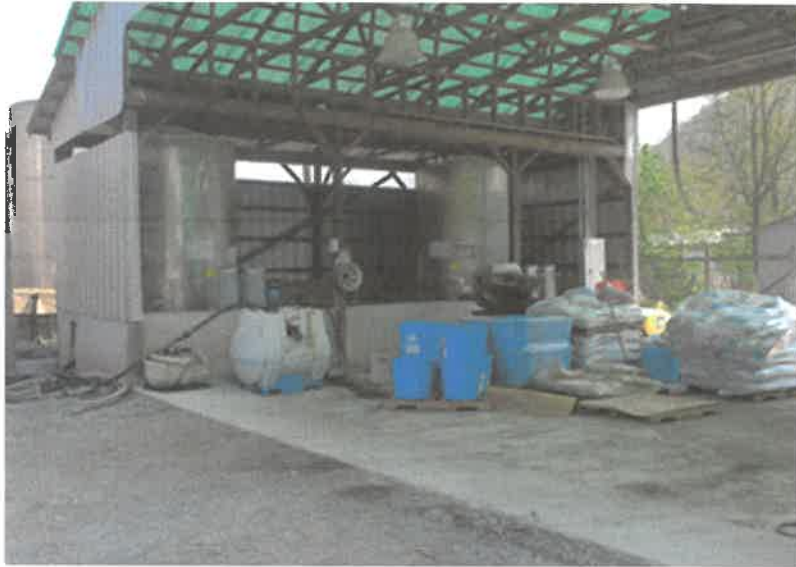
Secondary containment at a bulk facility.
