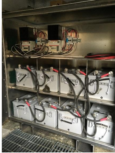
Figure 2: Battery box and electrical controls
