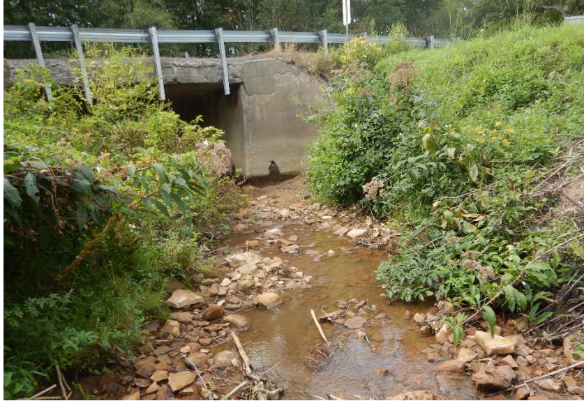
Figure 15. MRM site during low flow conditions on 7 Sept 16. Doser operational.
