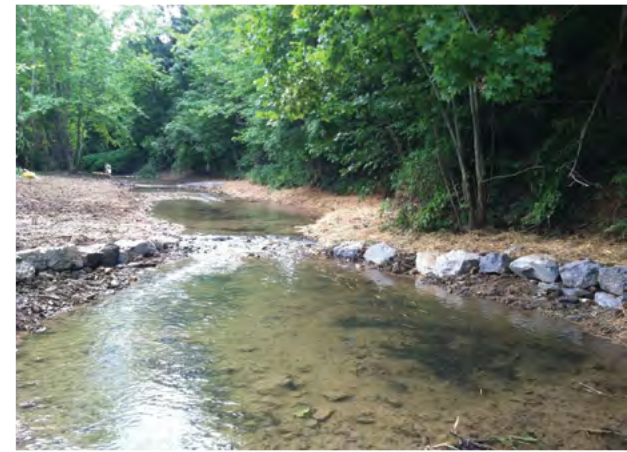
In the top picture, an area of Aaron's Creek had been over-widened due to a failed culvert upstream. As a result, a large mid-channel bar formed and divided the stream flow. In the picture on the bottom, it shows the same area with the bar removed and a cross-vane installed. The dirt from the bar was used to construct the bankfull benches on both sides of the stream.
