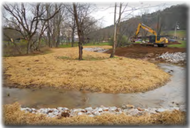
The Lewis County Park Stream Bank Restoration Project cost $47,080, and benefits many local residents and organizations.
