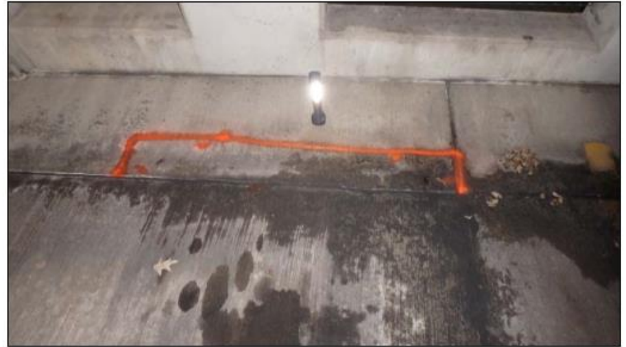
Photograph 2: Delaminated Concrete Locations
