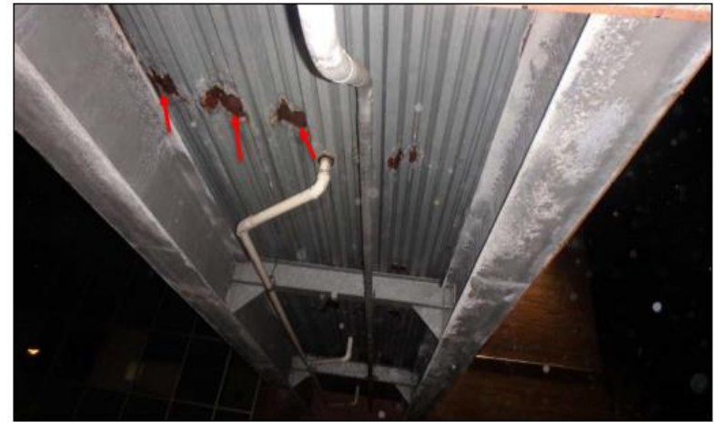
Photograph 23: Corroded Metal Deck at Bridge Underside
