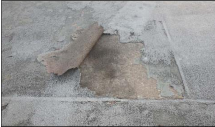
Photograph 16: Damaged Traffic Bearing Membrane
