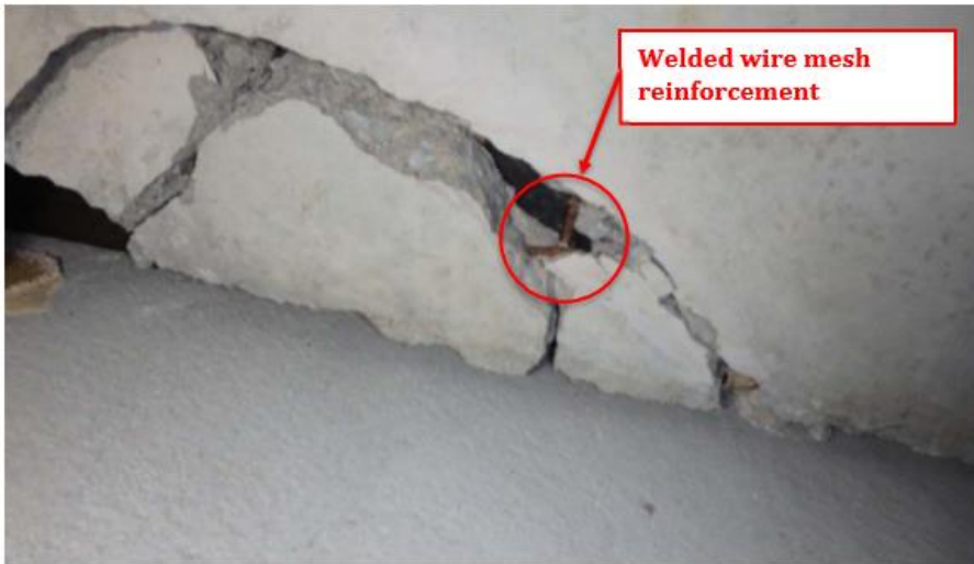
Photograph 7: Welded Wire Mesh at Fractured Flange
