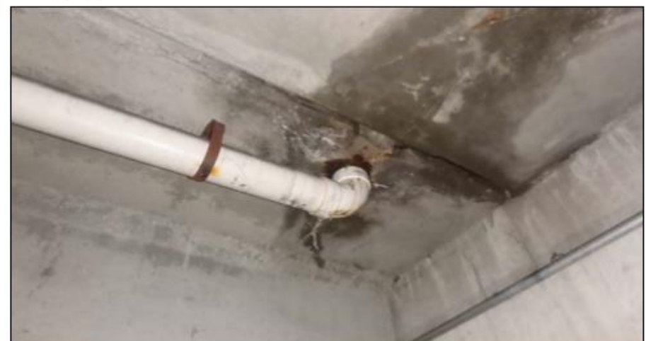
Photograph 13: Concrete Deterioration at Drain
