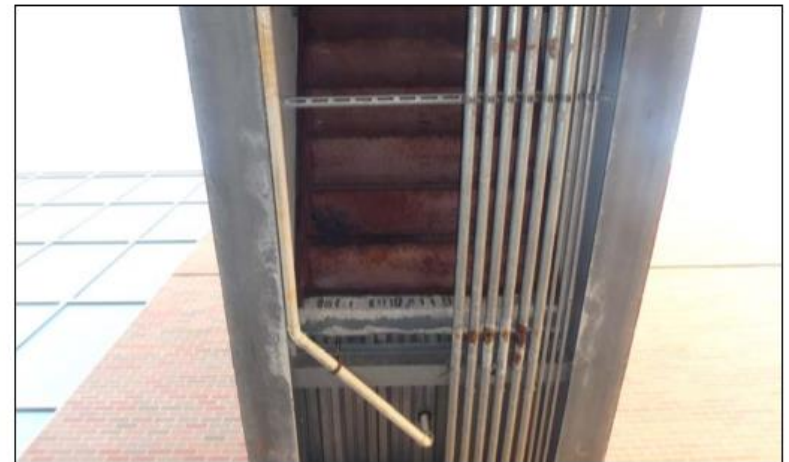
Photograph 24: Corrosion at Bridge Stairway
