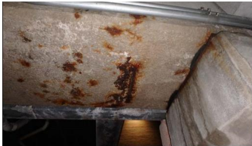
Photograph 8: Heavy Corrosion at Concrete Beam
