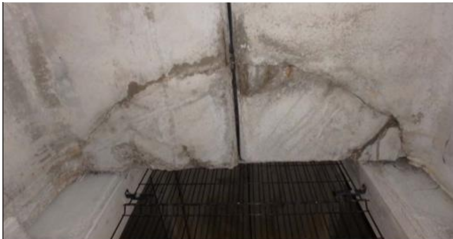
Photograph 5: Fractured Corners at Double Tee Flanges
