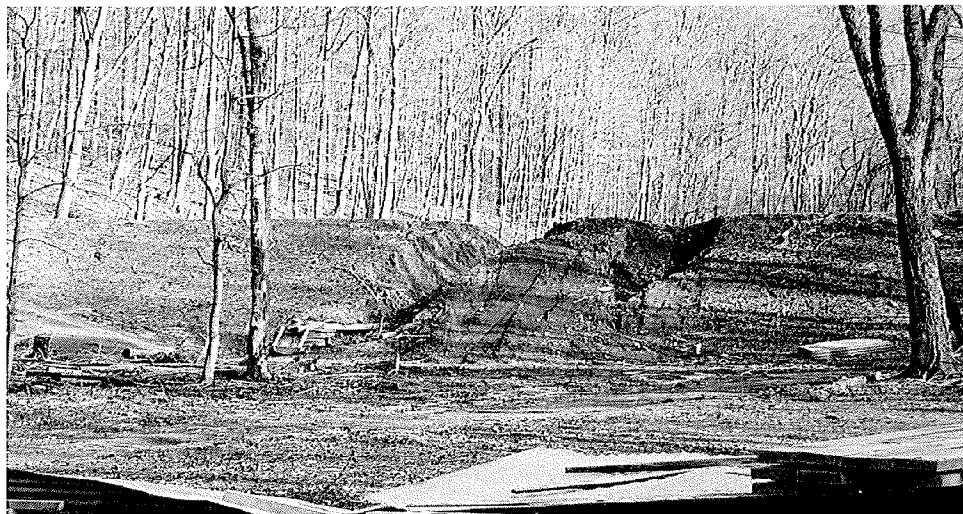
Image 1 Overtopping at Wetzel County Dam
