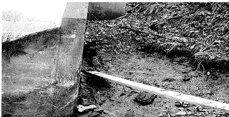
Image 2 Erosion from Seepage at Lake Washington
