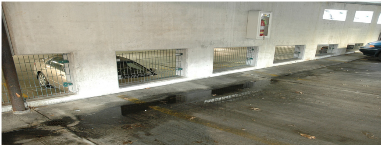
Figure 3 - Water pooling on garage floors as shown in the May 2006 report.
