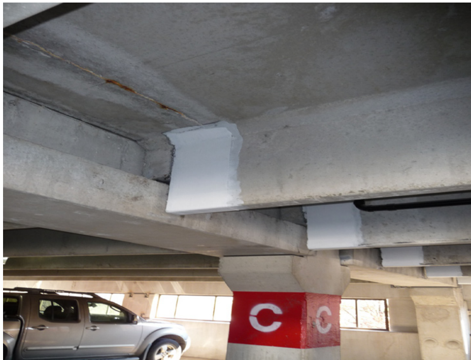
Figure 10 - Carbon fiber wrapped double tee precast beams to reinforce damaged precast concrete.
