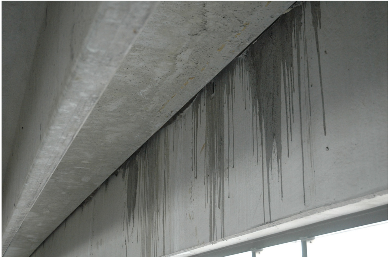
Figure 2 - Water leakage from the roof of the garage as photographed for the May 2006 report.
