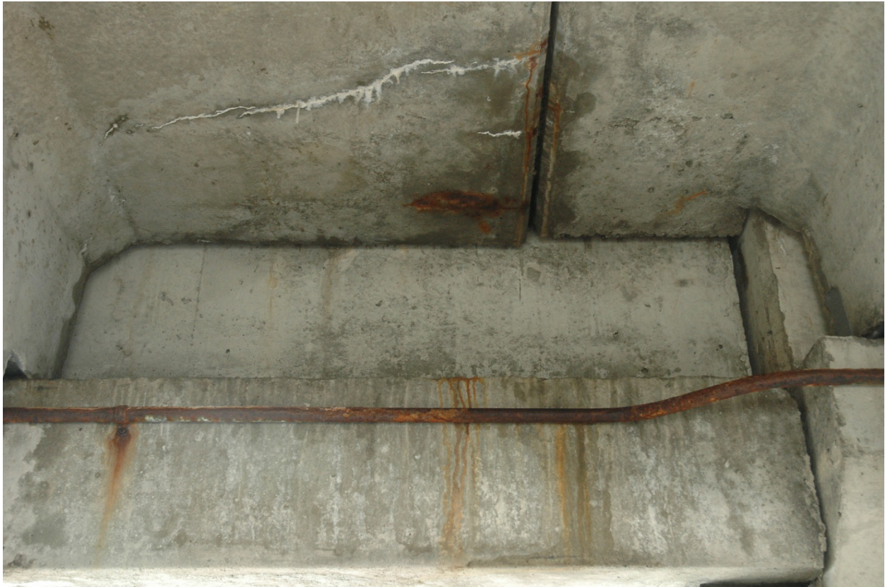
Figure 6 – Rusty electrical conduit as photographed for the May 2006 report.
