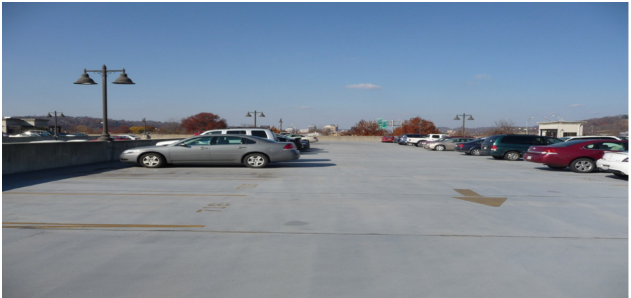
Figure 4 - A new roof deck coating has been applied to prevent water penetration.
