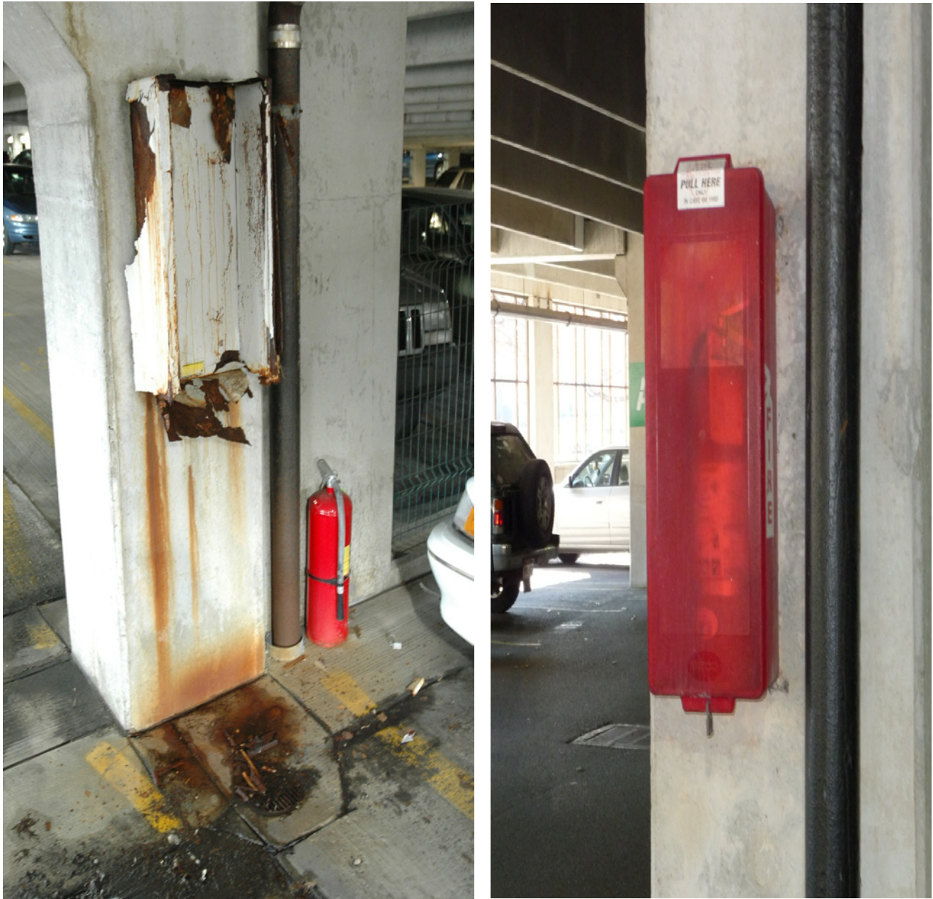
Figure 1 – At left, rusted fire extinguisher cabinet as presented in the May 2006 report. At right, new fire extinguisher enclosure to replace deteriorated metal cabinet.
